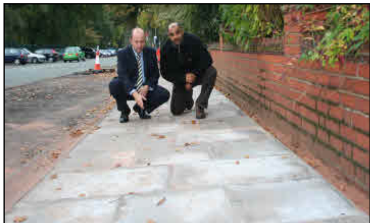
Left: Park Road East resident, Mr Bhuphinder Masaun, shows Cllr Robin Lawrence a completed section of new paving
