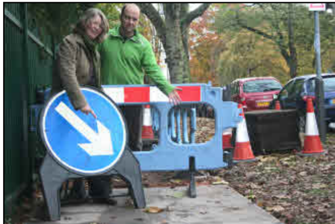
Cllr Claire Darke and Cllr Robin Lawrence were delighted to see these new paving slabs being put down
